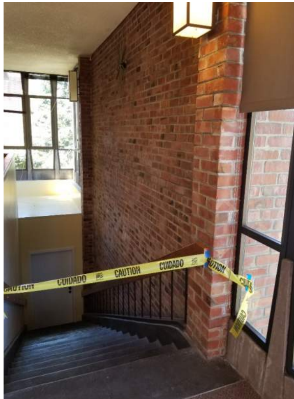
Large stair opening in the diaphragm at First Floor next to the exterior shear wall causing a two story wall
