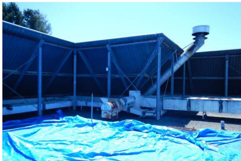
Roof screen at roof perimeter with a mechanical well in the center
