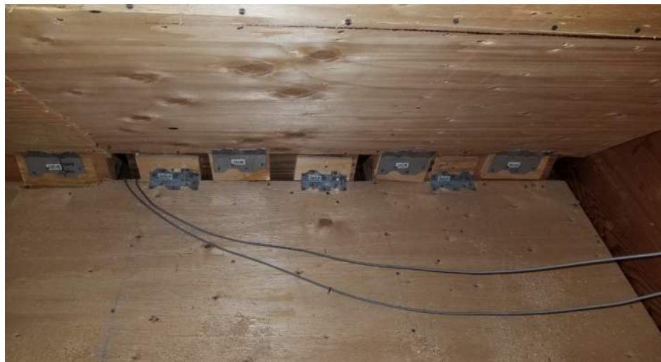
Retrofit at Attic and Roof showing new plywood sheathing and A35 connectors
