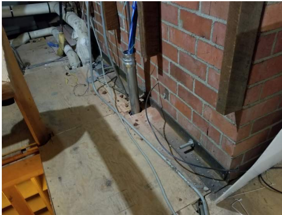
Shared masonry wall between Johnston Hall and Library Stacks with diaphragm connection with steel angle
