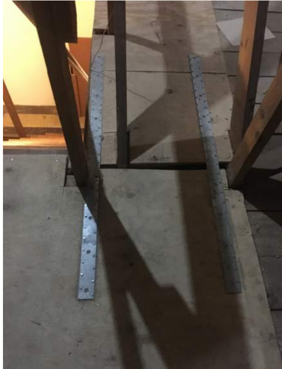
Retrofit at Attic showing new straps on plywood diaphragm near stair opening
