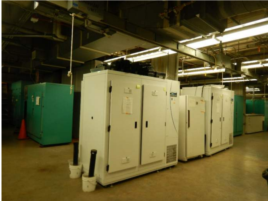
Figure A.3 Unanchored heavy cabinets
