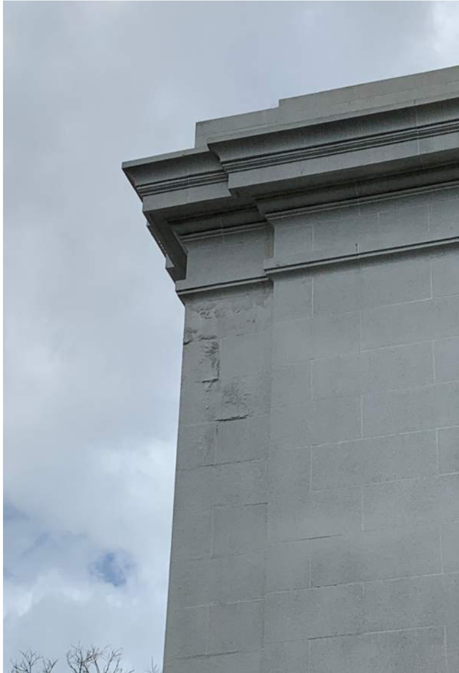
Figure 3 Terra Cotta deterioration
