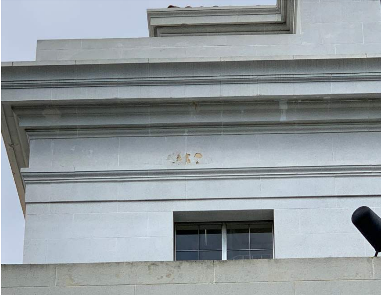
Figure 2 Deterioration in the Terra Cotta facade
